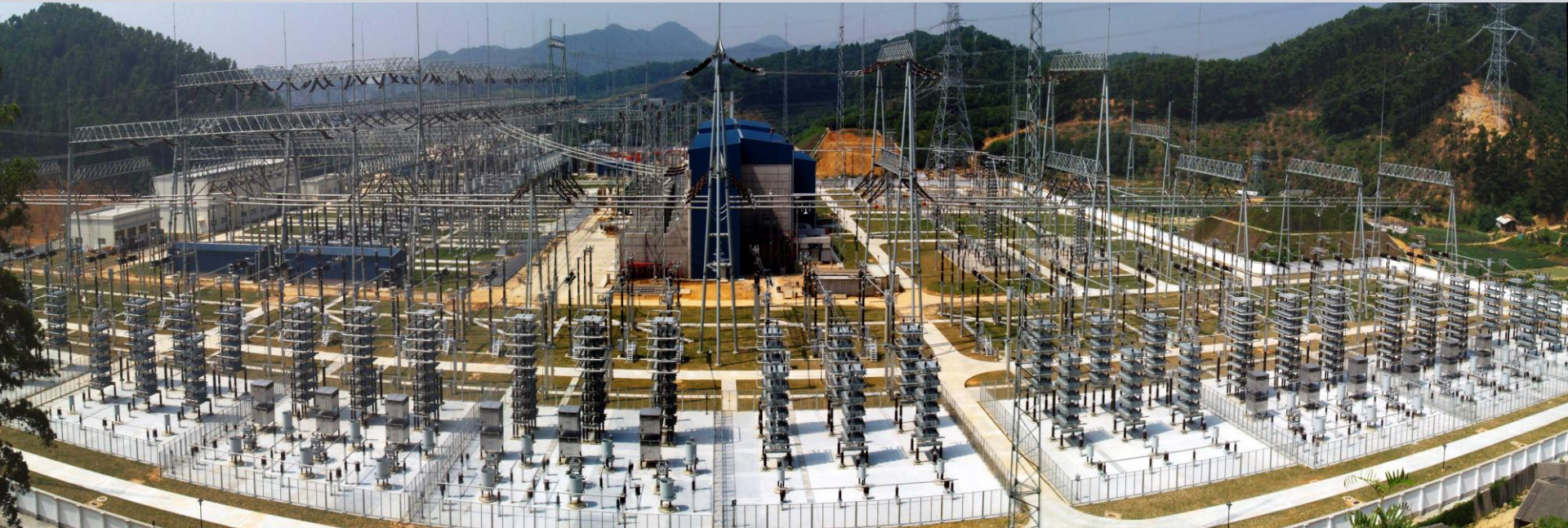
Shenzhen Converter Station (500 kV, 3000 MW) – HVDC LDT Guizhou-Guangdong II, China
