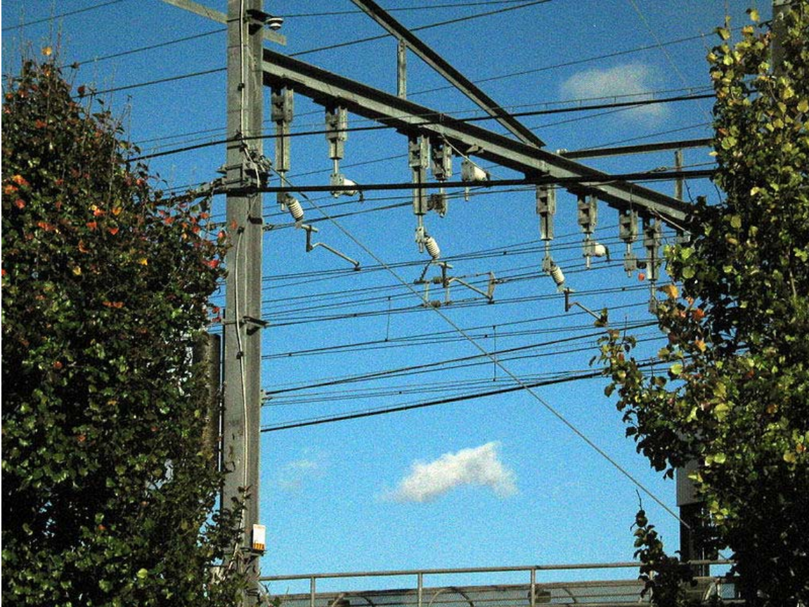
Close-up view of catenary on Northeast Corridor, United States
