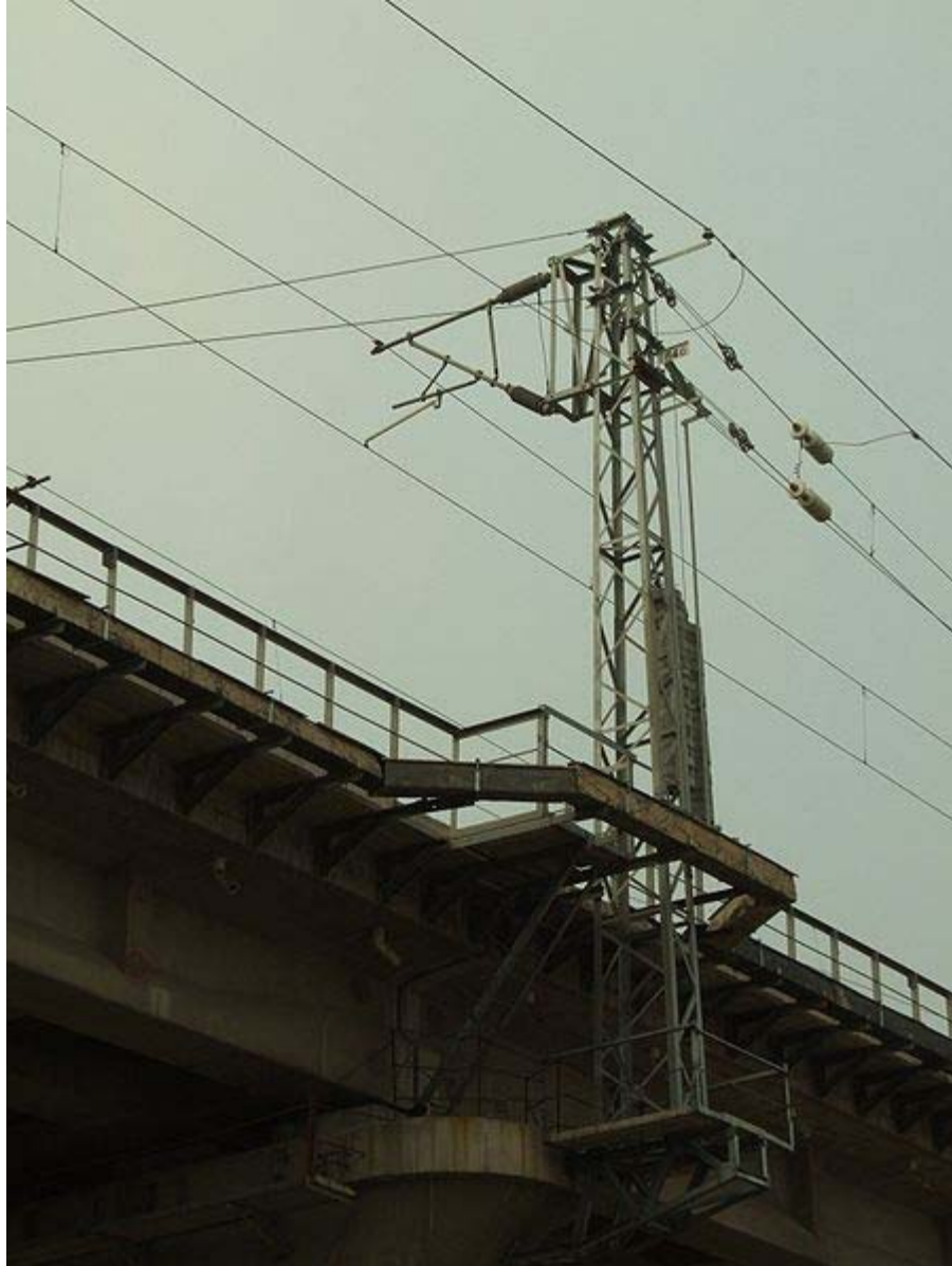
The overhead lines in China
