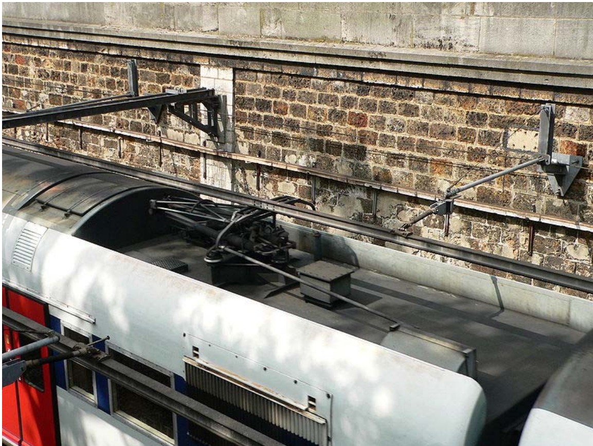
Overhead feeding rail on the RER Line C trenches and tunnels in central Paris
