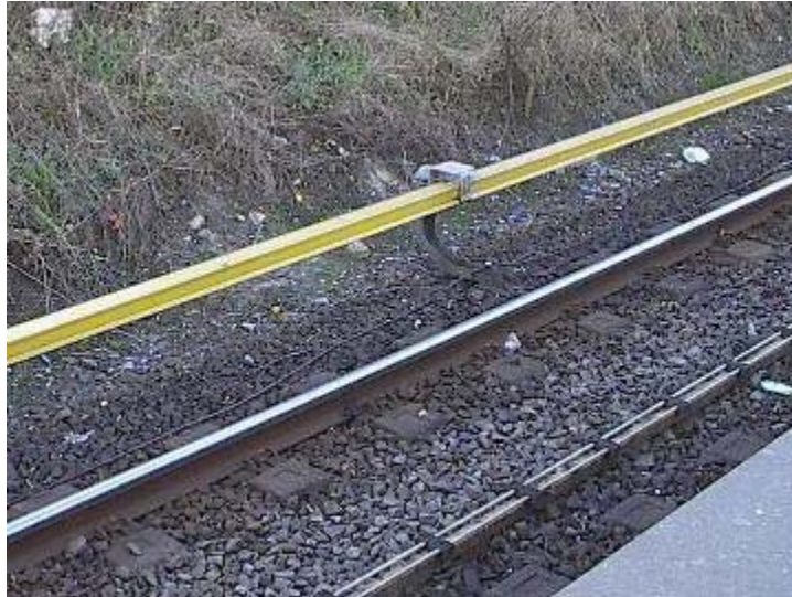
A bottom-contact third rail on the Amsterdam Metro, the Netherlands
