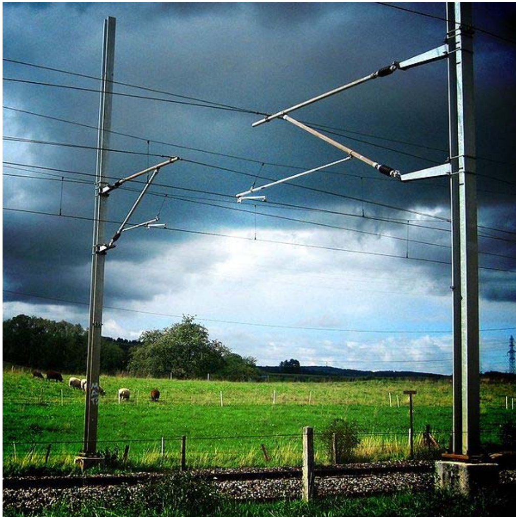
Overhead lines on Swiss Federal Railways
